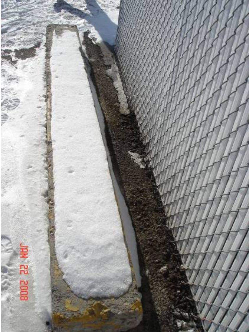
Neptune Engine Test Stand: Stormwater runoff controls off the engine test pad do not appear to fully direct stormwater to the underground oil/water interceptor; some staining of soil was evident.
