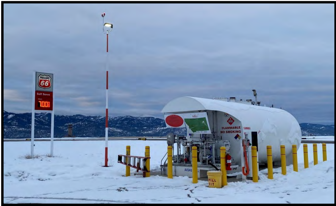
Northstar Self-Serve Fuel Station
