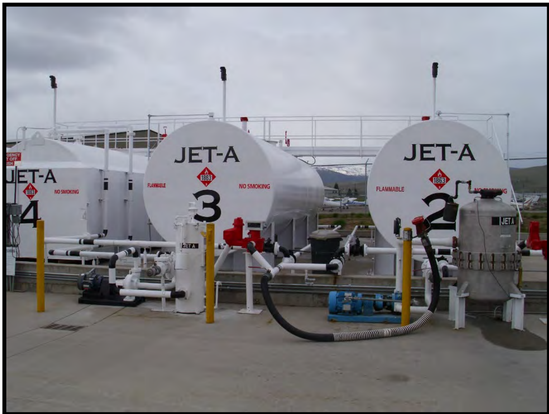
Fuel Farm – Northeast corner of Airport Property
