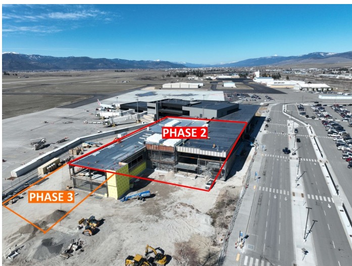
The new terminal construction continues in phases. Phase 1, the "South Concourse" has been completed. Work on phases 2 and 3 is underway. Graphic by Tim Damrow.
